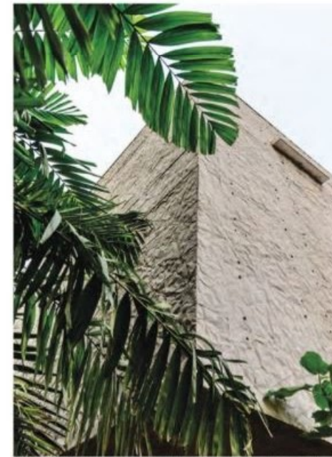
1 The shell of the house and much of the interior is constructed in form finished concrete.
